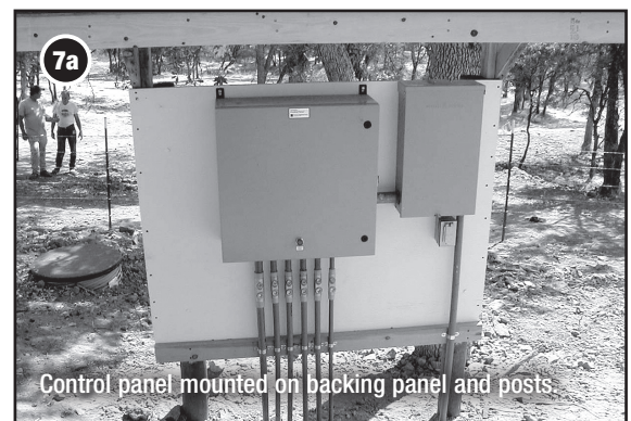
Control panel mounted on external wall.
