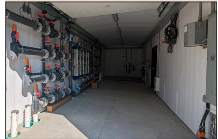
The UV units, plumbing, and valving came preinstalled in the wastewater utility building, along with the chemical feed plumbing and flow meters.
