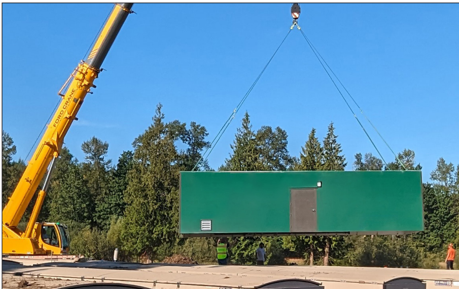
Weighing 12,000 pounds and 10,600 pounds (5443 and 4808 kg), the two DuraFiber buildings were installed in just four hours: lifted by crane, set on concrete, and attached with anchors.
