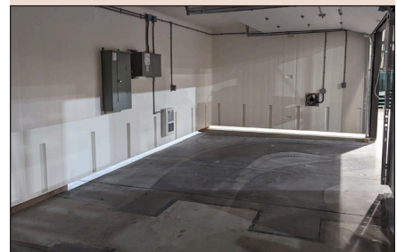
The two-room water utility building has preinstalled wiring and electrical panels that operate pump skids and chemical feed equipment.
