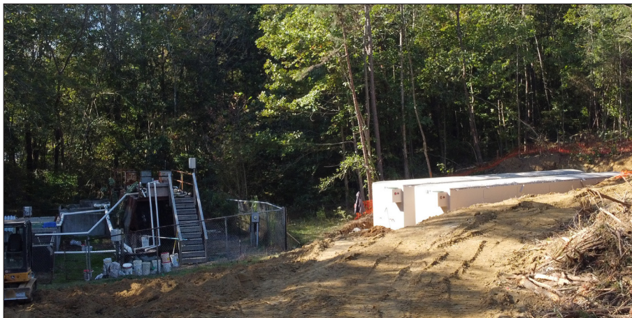
Because the AdvanTex AX-Max Wastewater Treatment System has a small footprint, these units (at right) could be installed while the old plant (at left) was still operating.
