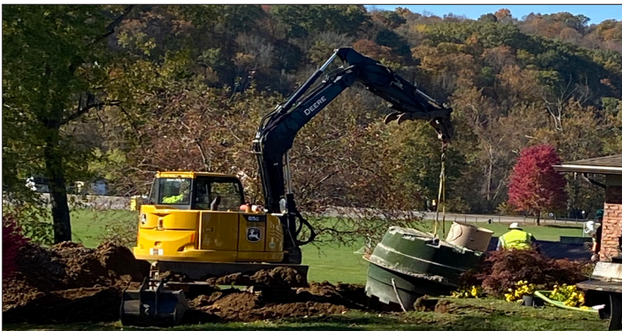
Despite a tentative decision for grinder sewer, county leaders changed course after comparing costs and ultimately chose an Orenco Prelos Sewer. The project went from concept to construction in less than a year.
