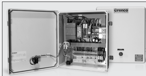
MVP control panels are used to control single pumps and provide alarm functions in on-site pumping systems.
