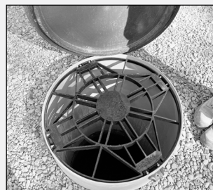
Secondary safety barriers fit securely inside access risers.
