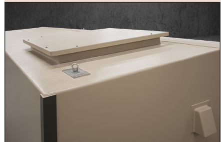
The two-room water utility building houses the water system's booster pumps. It has a custom hatch on the roof for easier pump removal.
