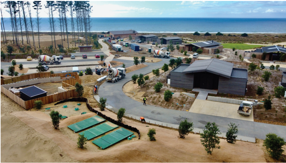
In Tomarata, New Zealand, 17 tourist cottages are served by an AdvanTex AX100 Wastewater Treatment facility that produces effluent clean enough to be discharged into the local sand hills. More than 55,000 AdvanTex units have been installed around the world. Photo courtesy of Innoflow.
