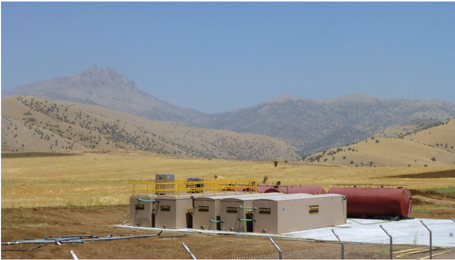
A seismic surveying firm needed portable wastewater systems for a series of remote camps in Iraq. The AX-Mobile was chosen for its ability to meet treatment limits with minimal operation and maintenance needs.
