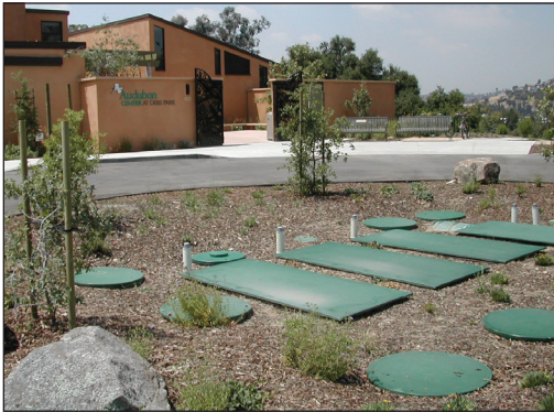
The Audubon Center’s AdvanTex Treatment System produces such high-quality effluent that it is reused for irrigation, and, when permitted, will also be reused for toilet flushing. Photo courtesy of BioSolutions, Inc.
