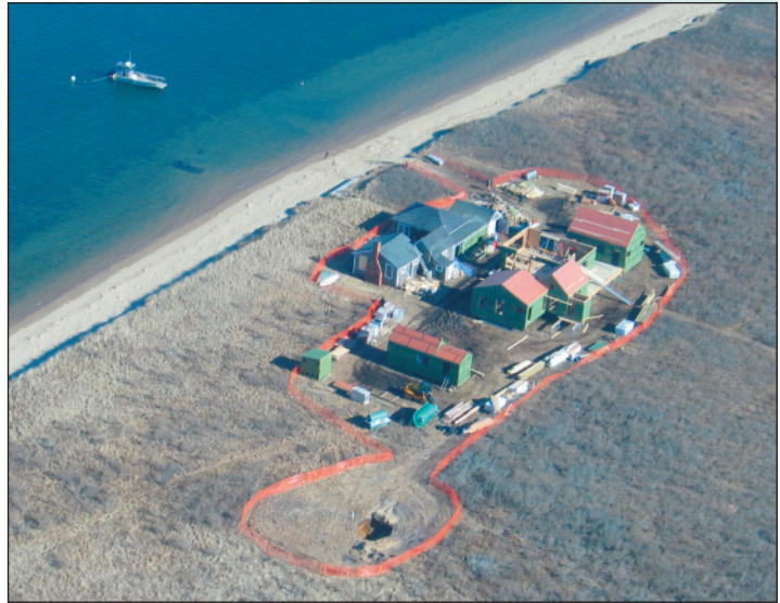
This aerial view of the Esther's Island construction site shows the protective fencing around the project perimeter and the green Orenco fiberglass tank, lying on its side, in the foreground. Photo courtesy of Tetra Tech Rizzo.
