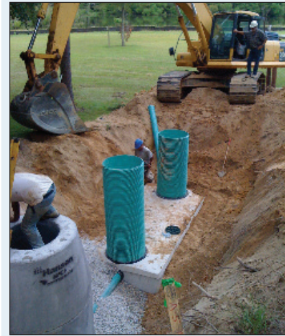
Effluent sewer technology can affordably link into existing sewer systems.
