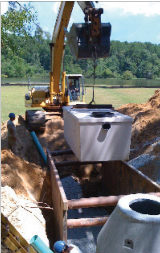
One 1500-gallon tank serves up to 5 or 6 campsites.
