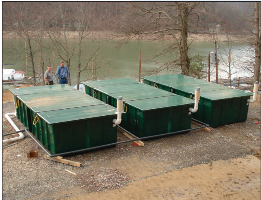
The AdvanTex pods were installed directly on top of the sand filter site.
