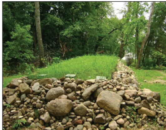
The existing drainfield on the east side of the house was replaced with a small, 300 sq ft box mound dispersal area.
