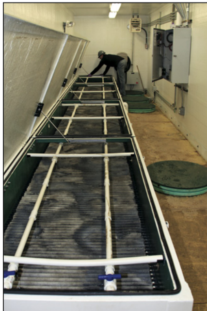
The insulated control room allows for easy maintenance regardless of weather conditions.
