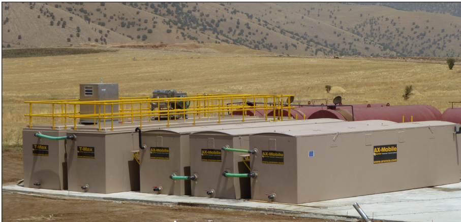
Portable AdvanTex AX-Mobile Wastewater Treatment Systems have been installed in remote areas of Kurdistan. They serve 500-person surveying camps.
