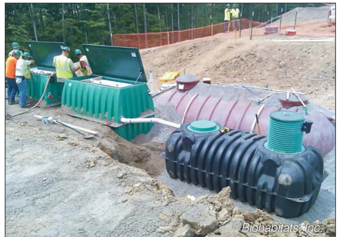
Treated greywater flows from the green AX20-RT units into the black dose tank and then to a UV disinfection unit. (The red tank in the background treats blackwater.)
