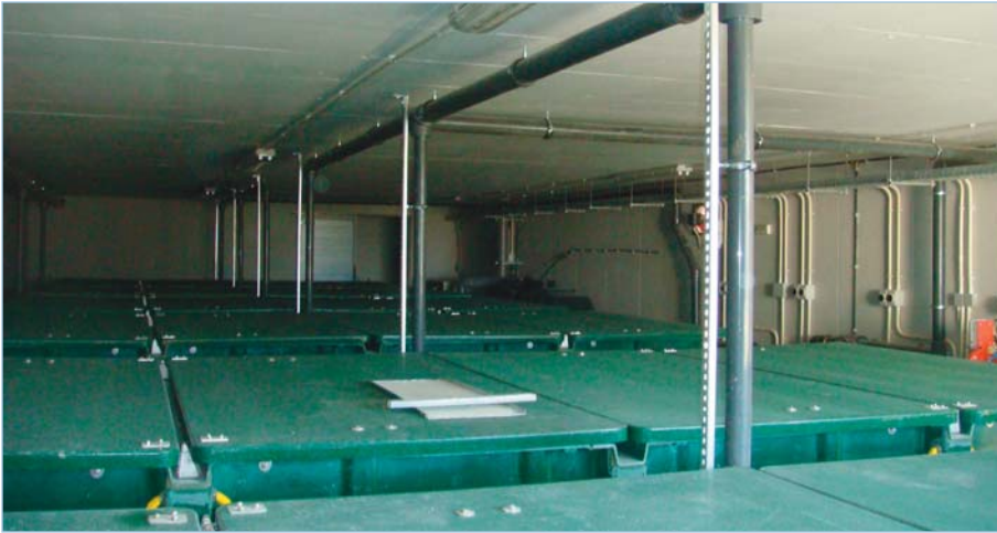
Following secondary treatment by six AX100s (pictured here), effluent flows through a sand filter for polishing and a chlorination unit for disinfection. It's then used for landscape irrigation.
