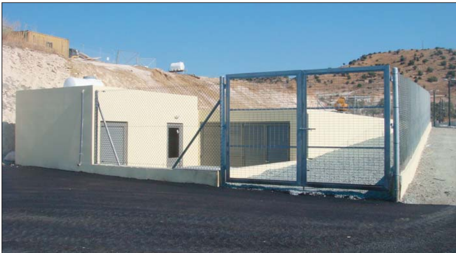
The AdvanTex® Treatment System is housed in this concrete building located directly above the septic, recirculation, and discharge tanks. Minimizing the footprint of the system was key to the success of this project.
