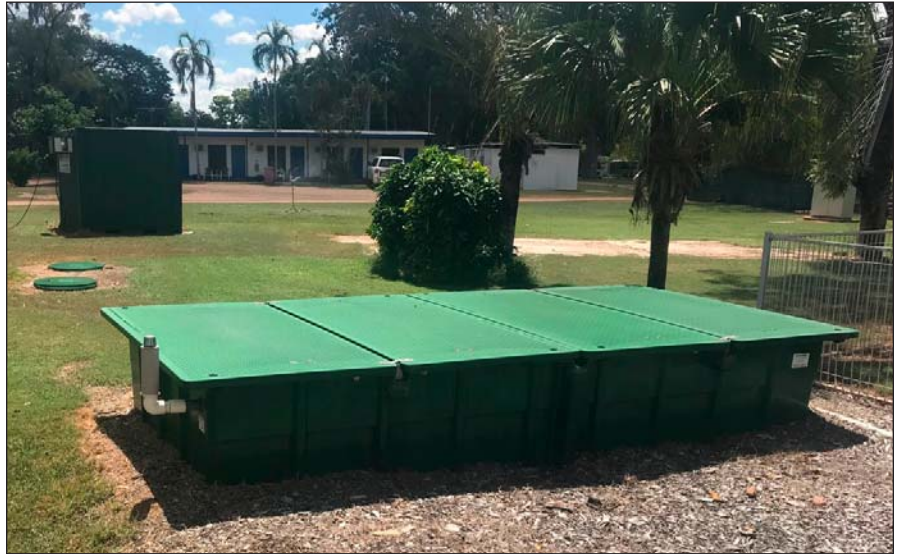
Because AdvanTex units can be installed in phases, the park will easily be able to expand its wastewater treatment capabilities in the future. Photo courtesy of ENVIRA Holdings.
