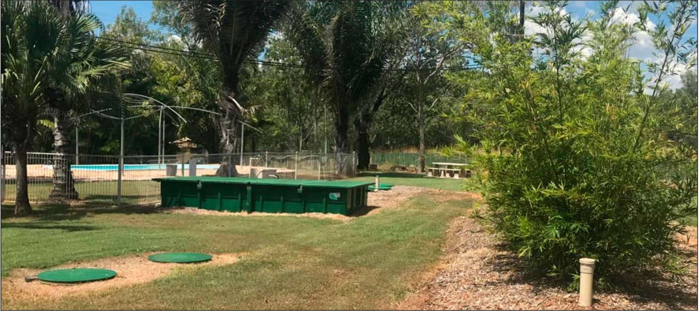
The AdvanTex system provides high-quality secondary wastewater treatment. Treated effluent is then dispersed through an ENVIRA Integrated Transpiration System, consisting of evapotranspiration beds (on the right) planted with select vegetation. Photo courtesy of ENVIRA Holdings.
