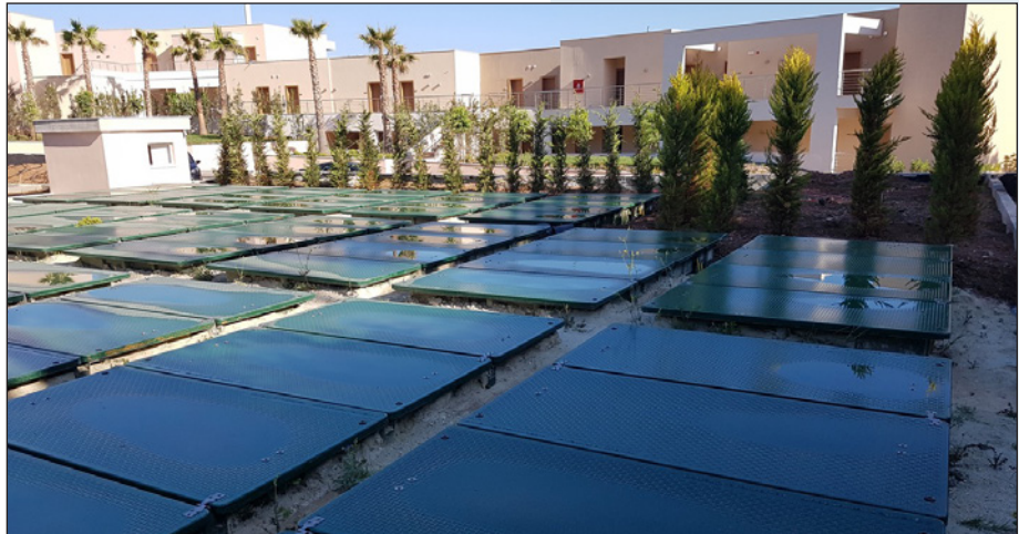
These twenty-two AX100s work around the clock, turning wastewater into high-quality effluent, which is then disinfected and reused for landscape irrigation.
