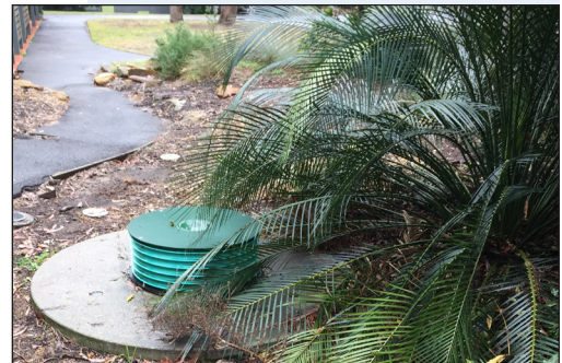
Tanks from the old treatment system were retrofitted with Orenco Biotube® pump packages and repurposed as septic tanks.
