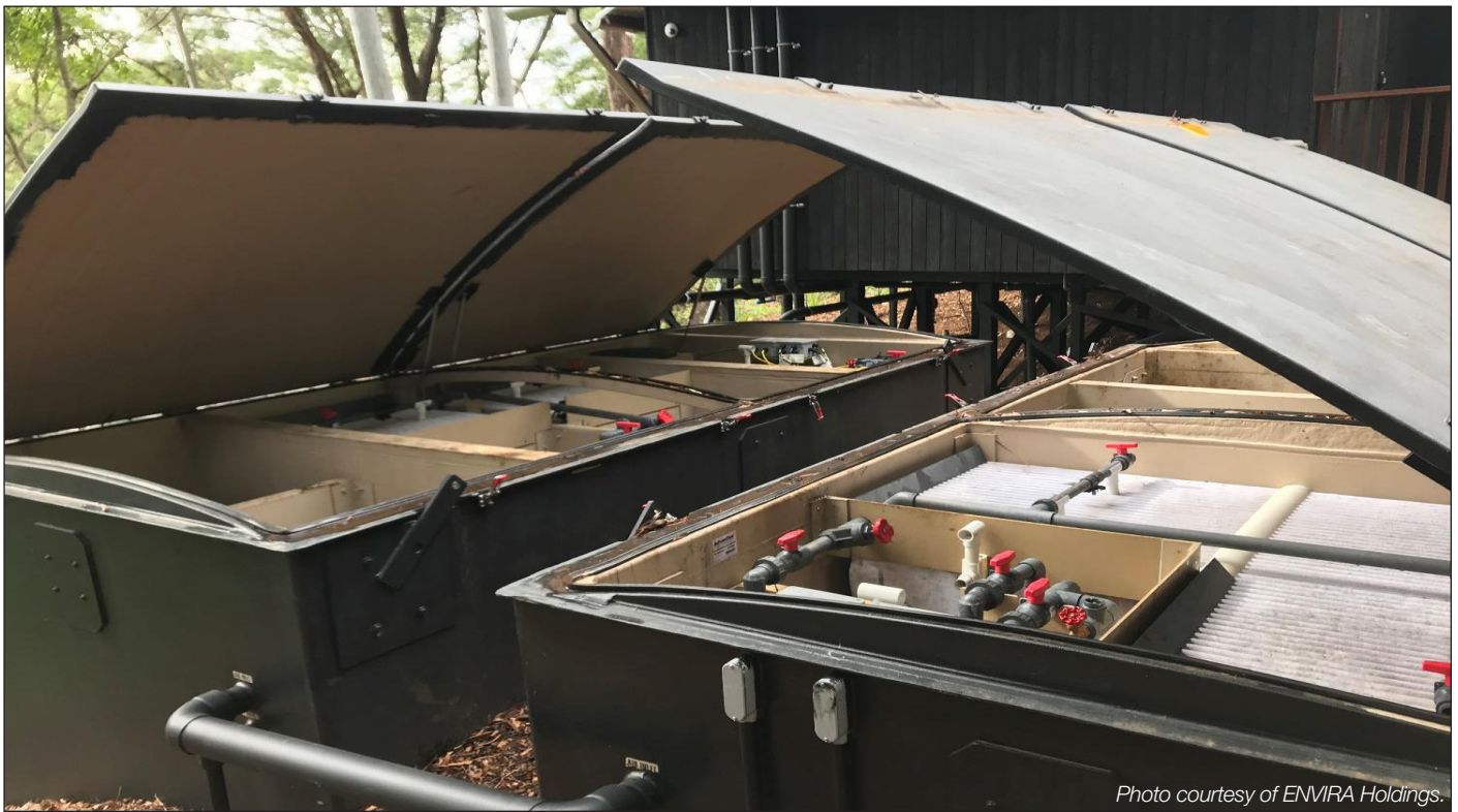
Photo courtesy of ENVIRA Holdings. These AX-Max units were custom designed to work together at this campsite. Integrated into the unit on the right is an 8300-L (2200-gallon) tank that's divided in half to accommodate both primary and pre-anoxic chambers.
