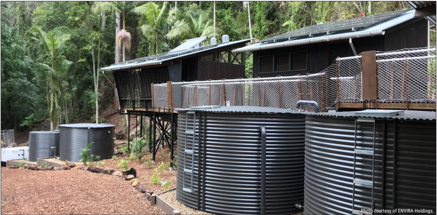
Treated effluent from the AdvanTex system is clean enough to be reused as subsurface irrigation. Left to right, the storage tanks at this off-grid camp contain treated AdvanTex effluent, rainwater for fighting bushfires, and rainwater that will be treated and used as potable water (two tanks).
