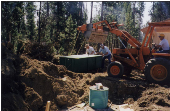
In La Pine, Oregon, an EPA wastewater demonstration project included six of Orenco’s AdvanTex Treatment Systems.
