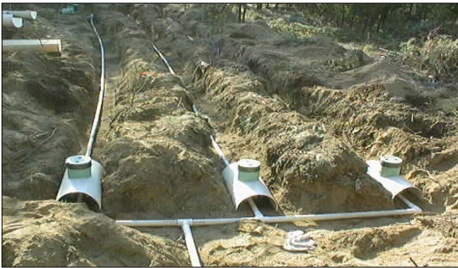
Treated effluent from one of the AdvanTex systems is dispersed through three shallow pressure lines totaling 105 linear feet (32 m).
