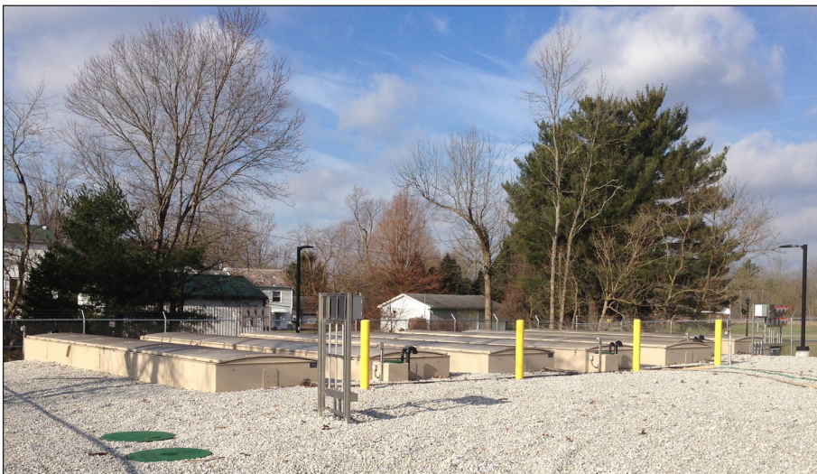
An Orenco Sewer collection system, followed by these AdvanTex AX-Max treatment units, was estimated to cost Lore City approximately $1.1 million less than a gravity sewer with a package treatment plant.
