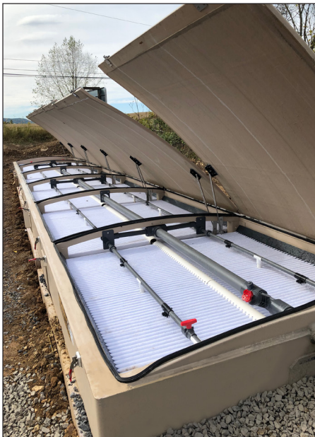
When complete, the Potters Mills AdvanTex facility can be expanded in four phases to handle the wastewater from up to 170 equivalent dwelling units.
