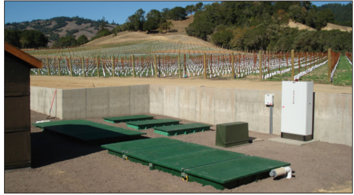
Jim Ball Vineyards in Mendocino, California, installed two AdvanTex AX100 units to treat processing waste from the winery and three AX20 units to treat domestic waste from the tasting facility.
