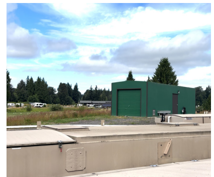
Angel of the Winds RV Park uses AdvanTex AX-Max and OmniMax-D systems to deliver advanced wastewater treatment and nutrient removal.
