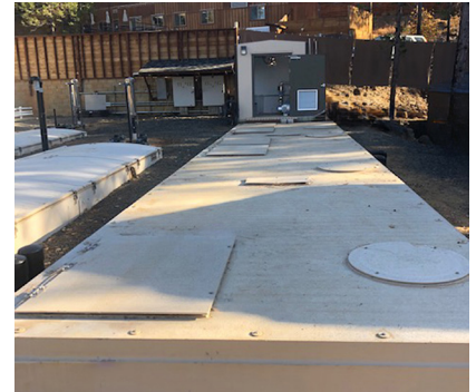
Orenco Controls™ and Orenco Composites™ (divisions of Orenco Systems) supplied the electrical control panels and DuraFiber utility buildings for this project.
