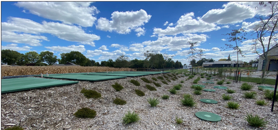
This AdvanTex Wastewater Treatment System is so quiet and efficient that it goes practically unnoticed by the residents of the Tamahere Country Club, a high-end retirement community.
