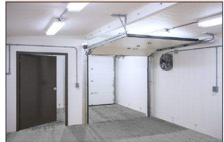
The wastewater building features two regular doors (one inside and one outside), as well as two overhead doors (one inside and one outside).
