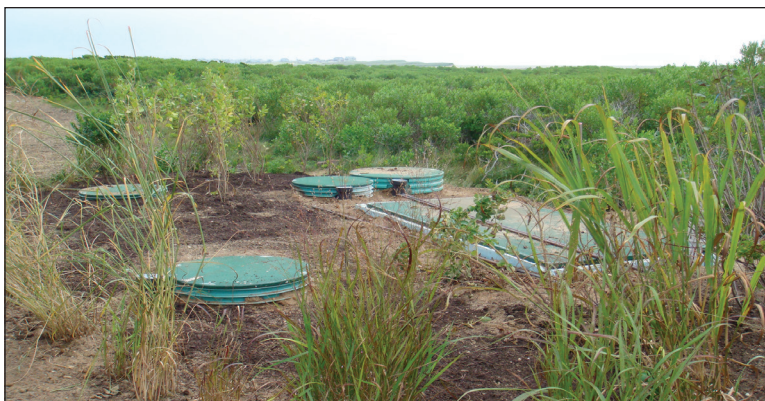
An Orenco AdvanTex® Treatment System nestles discreetly in the beach grass. This low-energy, highly reliable media filter replaced the former cesspool and treats this Esther’s Island household’s wastewater to reuse quality. Photo courtesy of Scout Capital.
