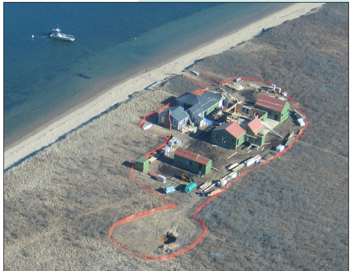
This aerial view of the Esther’s Island construction site shows the protective fencing around the project perimeter and the green Orenco fiberglass tank, lying on its side in the foreground.
